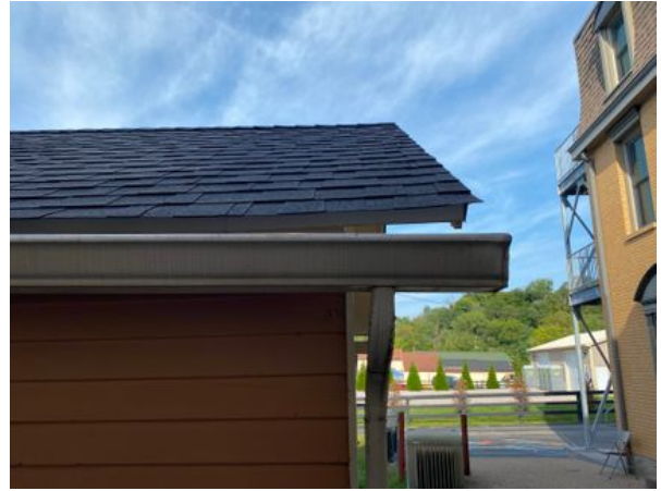
gutter needs repair
